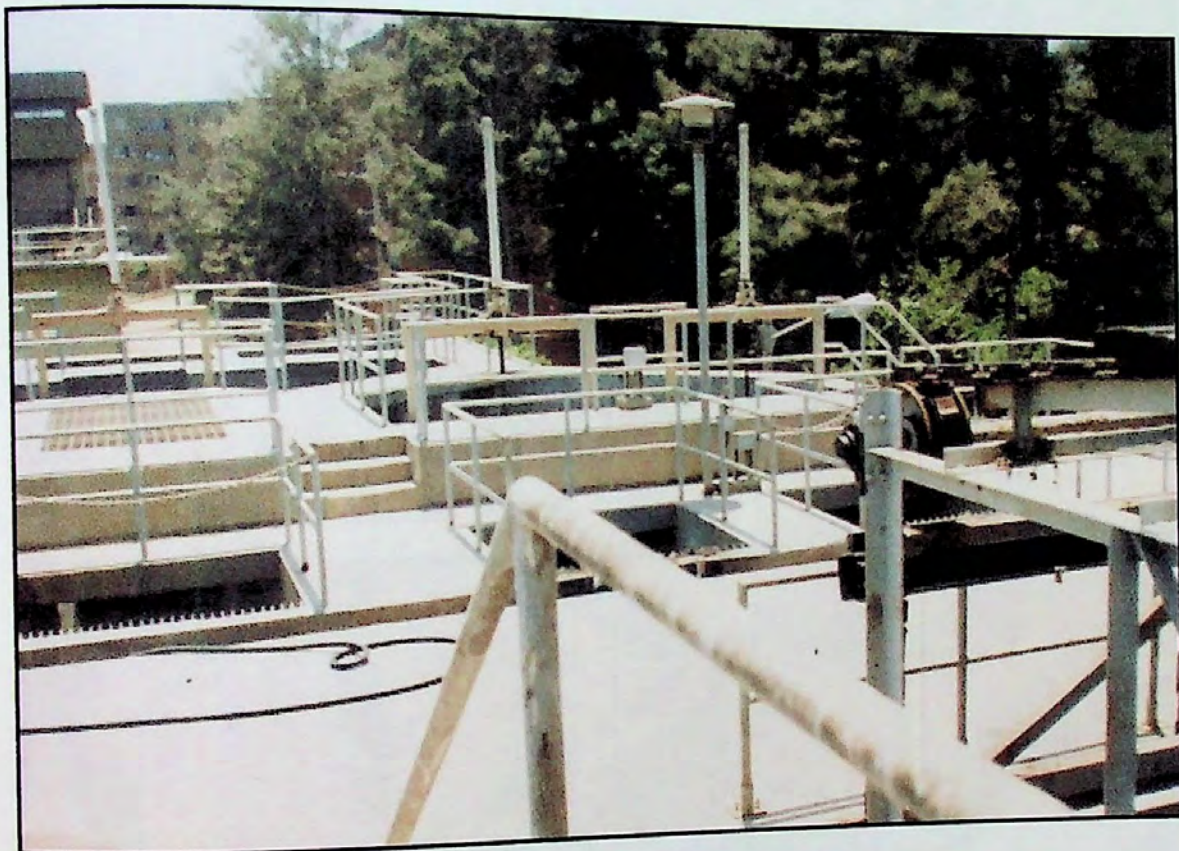
Fig. 39 : A) General view of the coarse manual screen
