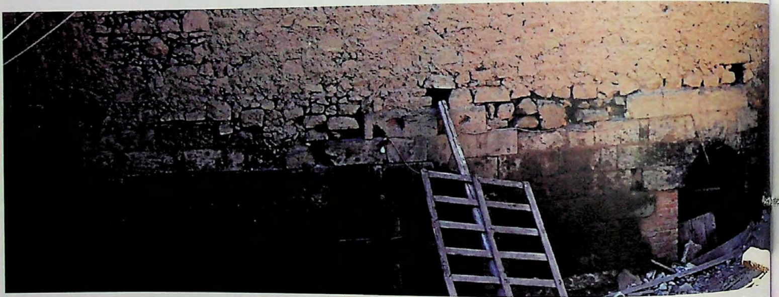
Figure 4.114. The rooms below the maq'ad with its four-pointed arched doorways and rectangular windows.
