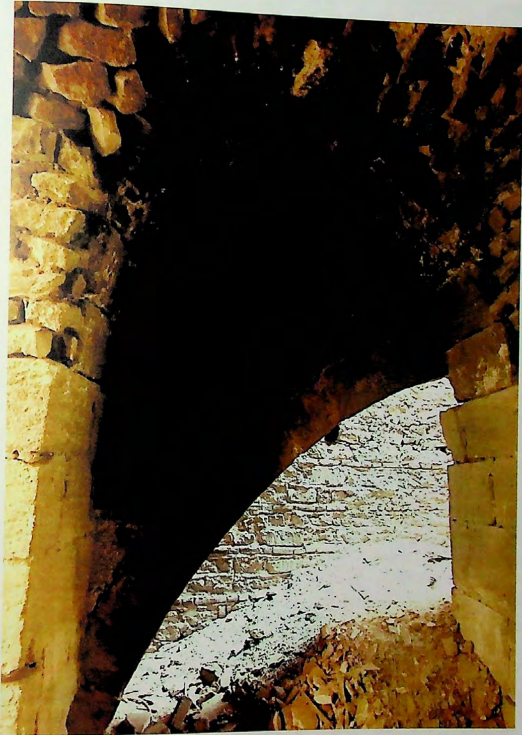
Figure 4.69. The arch that may have once opened up to the other parts at the southern end of the palace is interrupted by a massive pillar that nearly blocks its opening (no. 8 a on Plan E)
