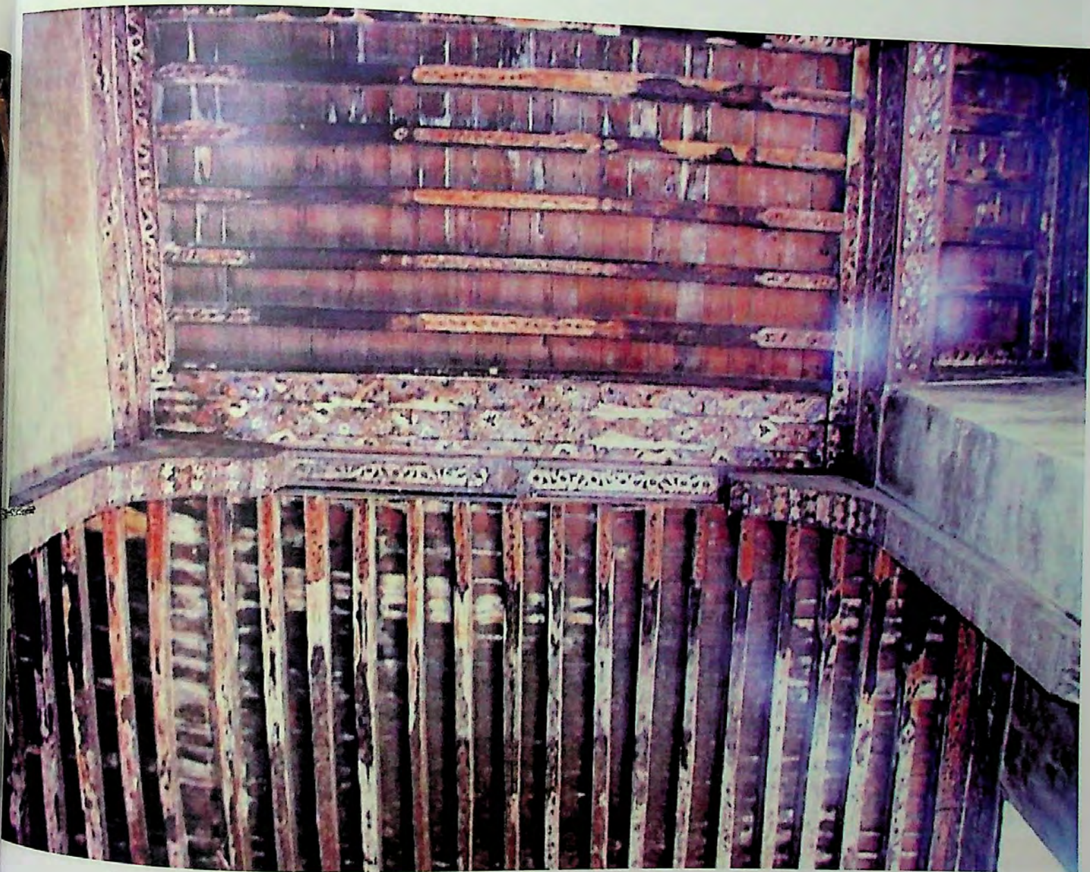
Figure 4.75. The ceiling of the qa'a in the first upper halls before parts of it collapsed (after Tavernari, L'évolution du Qasr Qawsûn-Yashbak ).
