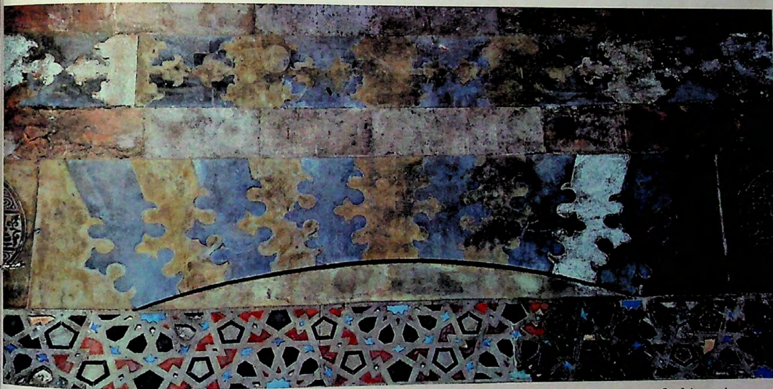
Figure 4.29. Detail of the joggled voissours above the entrance of the palace and the last traces of white paint. Above it is the marble frieze in black and white trefoils.
