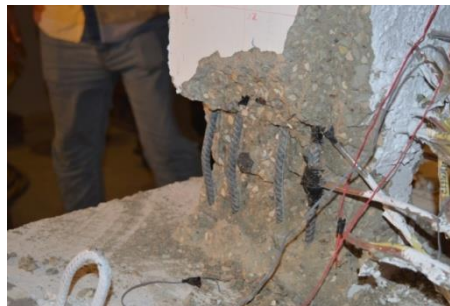
Figure 5.21: Compression side steel bars buckling
