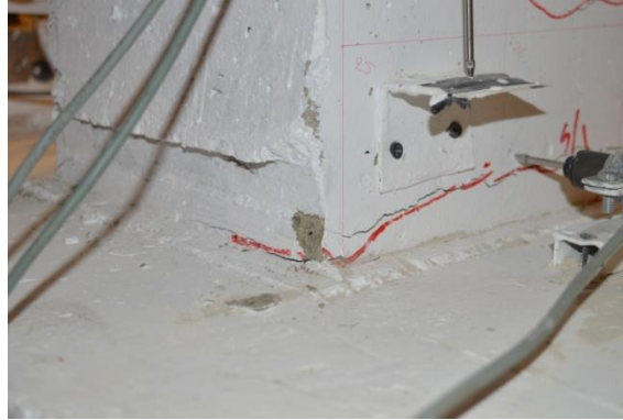
Figure 5.12: CSF-10-16-N slipping from base of column at 1.3\Delta y
