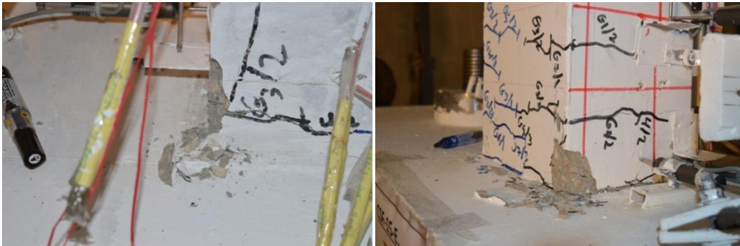
Figure 5.199: CSF-15-E crushing concrete cover at 1.69\Delta y
