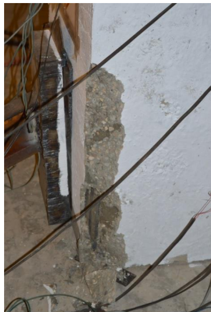
Figure 5.118: CSS-20-ECrushing concrete cover (2.85 \Delta y )
