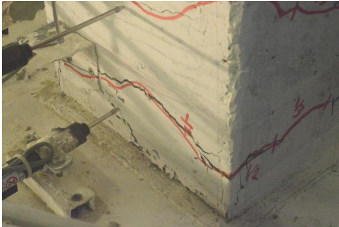
Figure 5.42: CSF-10-75 Boundary crack before failure
